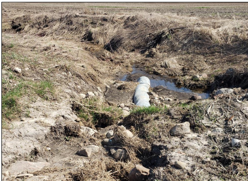
Figure 1- Bank slumping and erosion along the Main Drain (Open)
