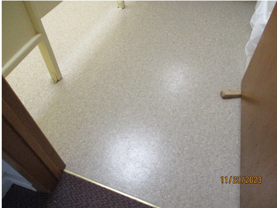
Photograph 1: View of non-asbestos linoleum in the Women's Washroom (Location 6) which is covering asbestos-containing vinyl sheet flooring, assigned a Priority 2 .
