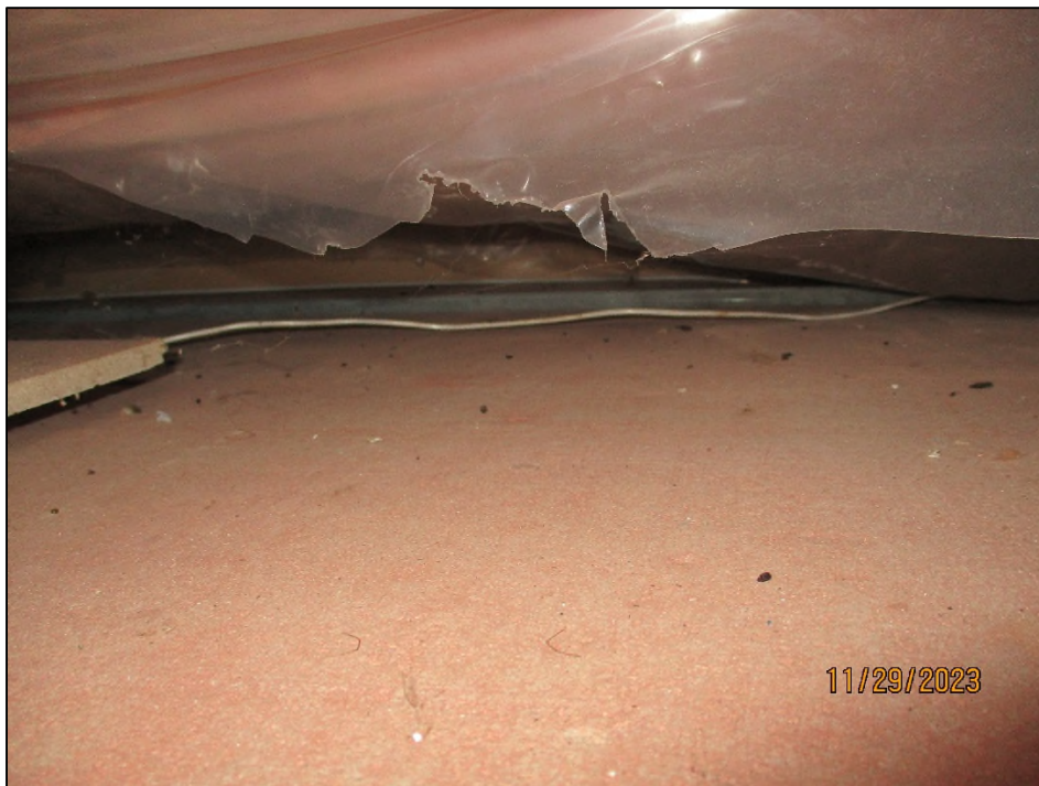
Photograph 4: View of mouse droppings on ceiling tiles in the Library Room (Location 2).
