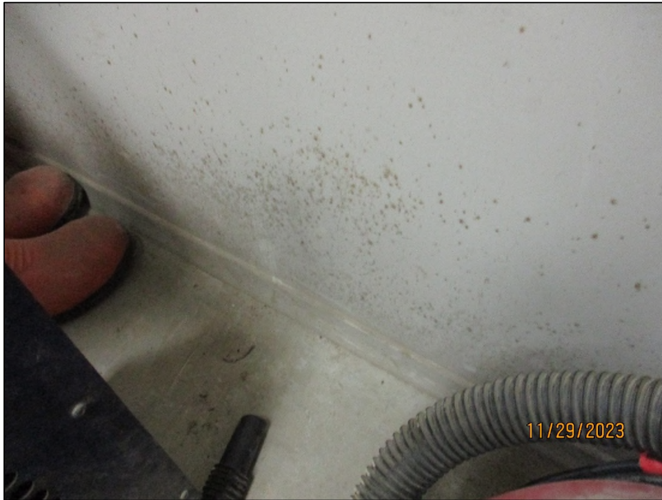
Photograph 1: View of suspect mould spotting on drywall walls in the Service Room.
