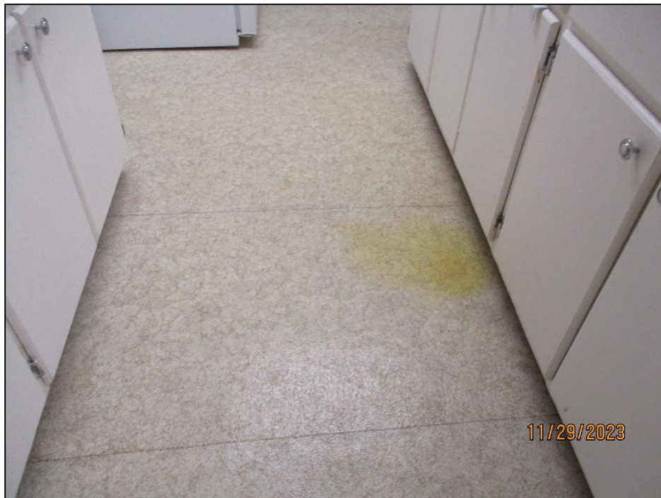
Photograph 2: View of asbestos-containing vinyl sheet flooring in the Kitchen (Location 7), assigned a Priority 2 .
