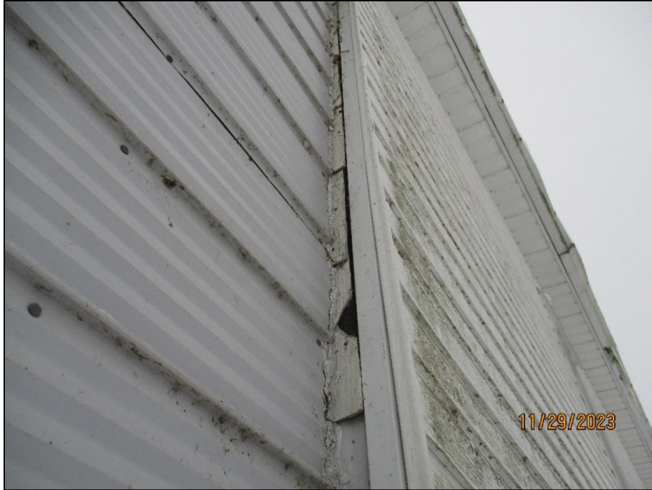
Photograph 3: View of asbestos-containing Transite Siding Shingles on the Building exterior, assigned a Priority 2 . No shingles were observed under the vinyl siding, where accessible, however, more shingles could be present under steel or vinyl siding.
