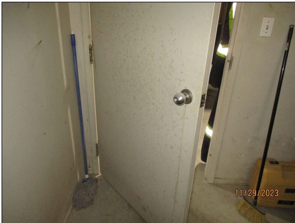
Photograph 2: View of suspect mould spotting on the wood door in the Service Room.
